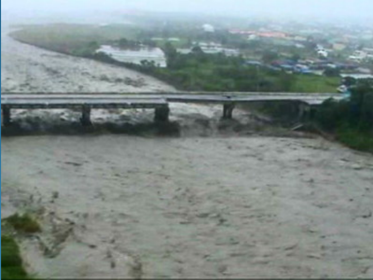
Bridge's failure due to high velocity flows
