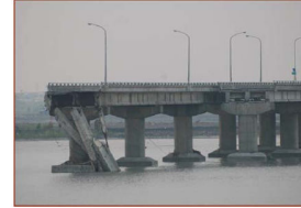
Fig. 18 Case 2: the bridge failure in flood
