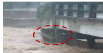
Fig. 19 Case 3: the bridge failure in flood
